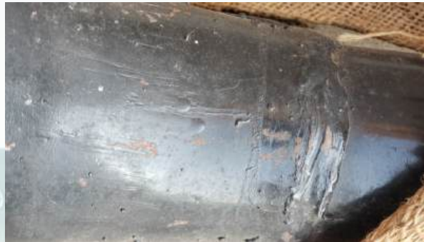
Close up showing paint runs
